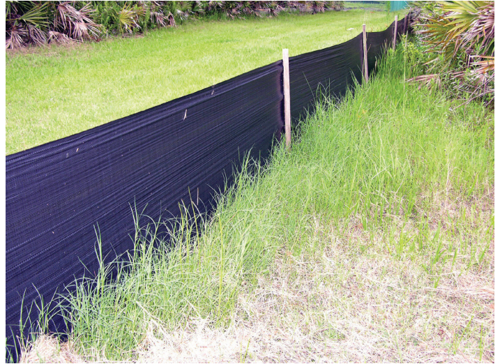
Figure 7. Snake fences, such as this one made of silt fencing, can prevent some snakes from entering your yard when used correctly, but can be costly and time consuming to install and do not prevent all species of snakes from entering. Such measures should only be used as a last resort.
