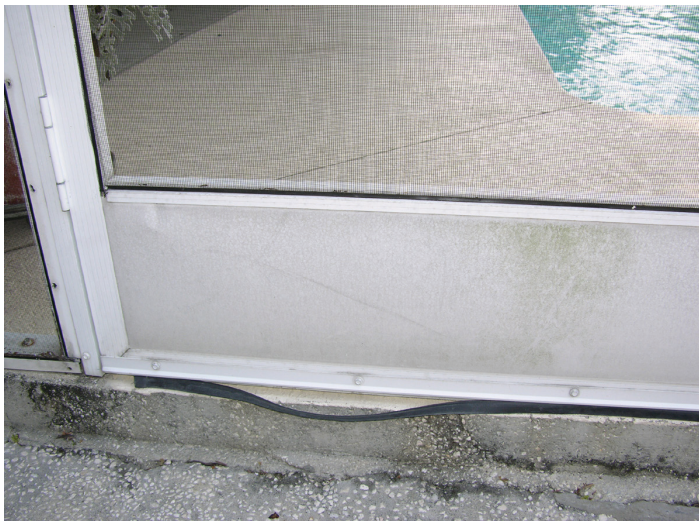
Figure 3. Door sweeps can prevent snakes from inadvertently slipping into the home under a door, but must be checked periodically. This rubber door strip is in disrepair, leaving large gaps beneath the door.
